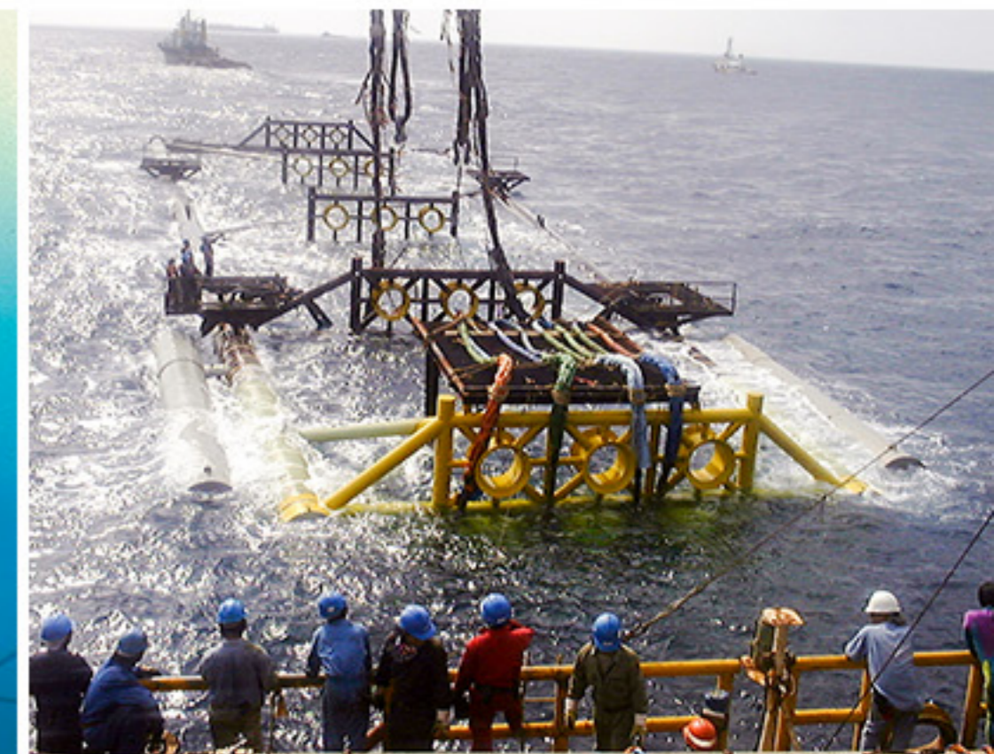
水深90mへの石油生産設備設置工事 Oil production facility installation in 90m water
